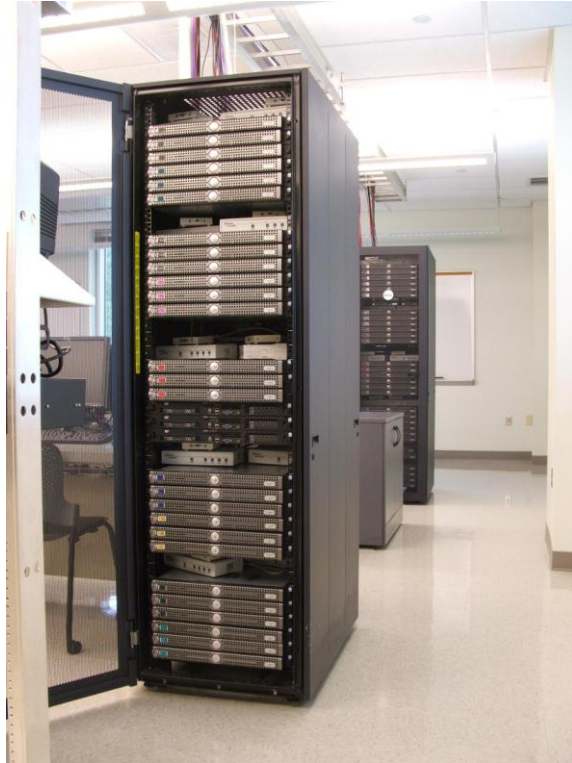
Illustration 5: Rack of 30 1-U servers. Note the boxes of KVM switches above each cluster of six servers. The bottom three servers in the middle cluster have their escutcheons removed to access their optical drives and USB ports.
