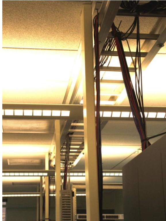
Illustration 4: The "ladder" carrying network cabling between rows of workstations. Note the bundle of cables rising obliquely from the server rack (right foreground) to the ladder, and vertical bundles of cables running from the ladder down to the trough below (not shown).
